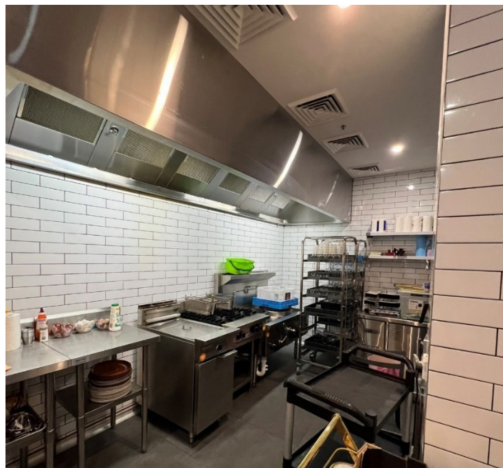
Figure 40 Industrial kitchen at 94 Hay Street.
